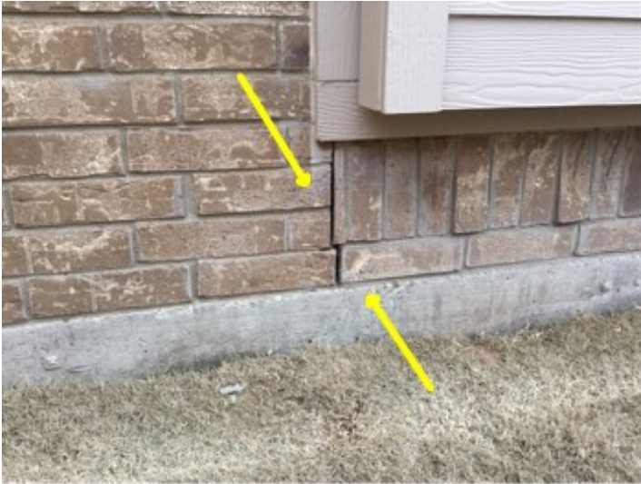
Large gap observed below window on west side of home
