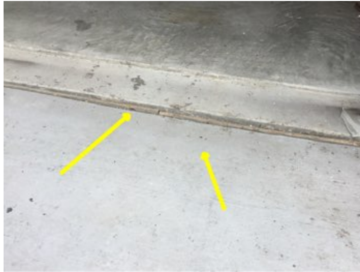
Trip hazard location between garage and driveway
