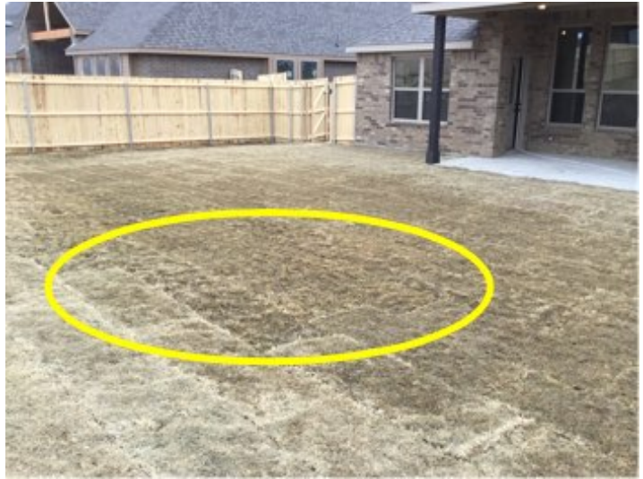
Excessive moisture observed in back yard, no drain installed
