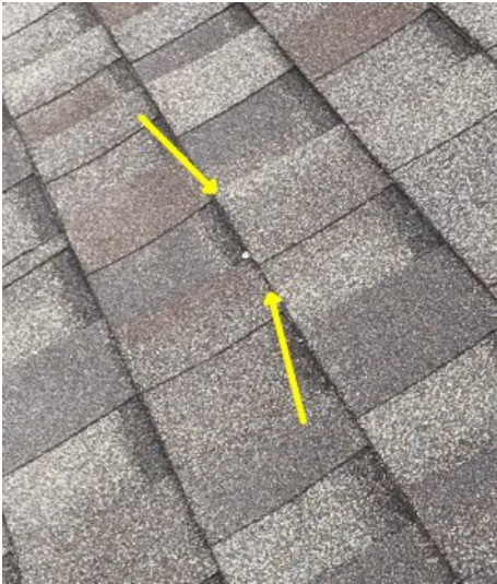
Exposed nails on shingles with sealant, could leak
