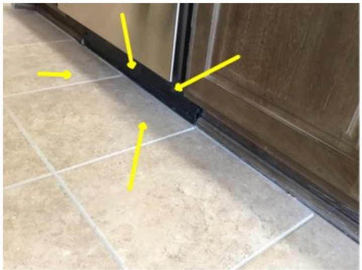
Gap between trim and tile beneath sink
