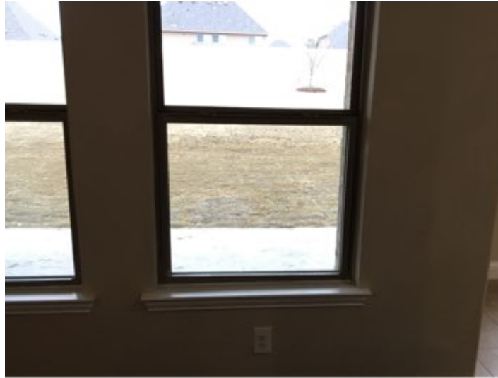
Some windows through house were difficult to operate, many need adjustments
