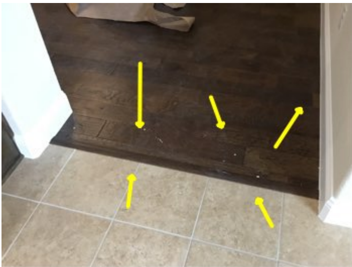
Spilled paint and overspray observed in many areas of the home
