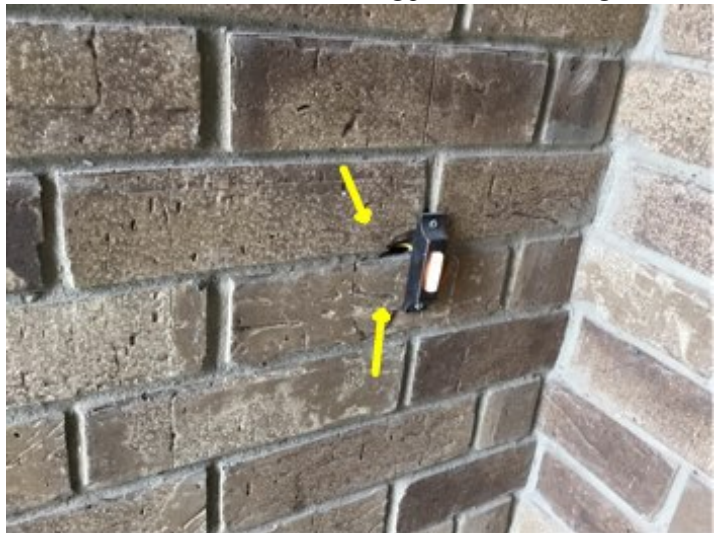
Hole around doorbell
