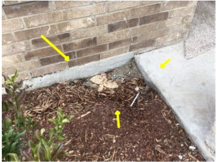
Washout from roof run off observed, gutters not installed
