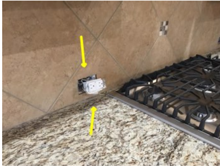
Missing outlet covers in kitchen and master bath
