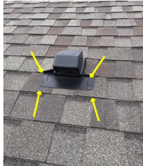
Unsealed nails on vents, could leak
