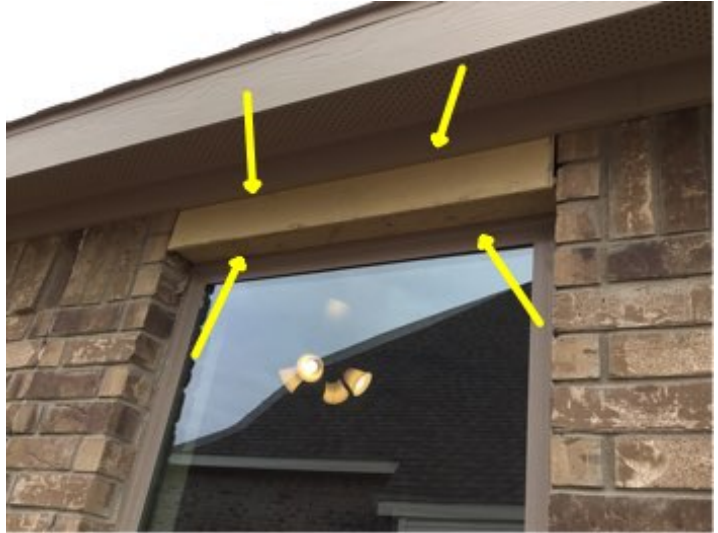
Area above window missing paint and caulking
