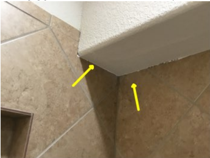
Missing caulk in master bath which could lead to moisture intrusion
