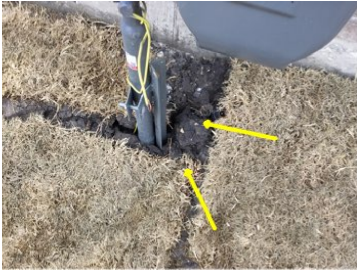
Loose and missing soil around gas meter causing irrigation pipes to be exposed
