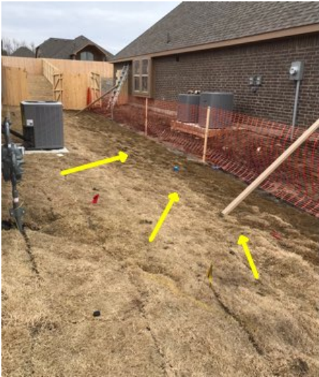
Excessive moisture located on east side of property
