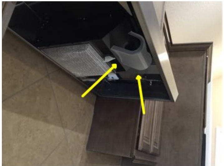
Missing bulb in stovetop vent fan
